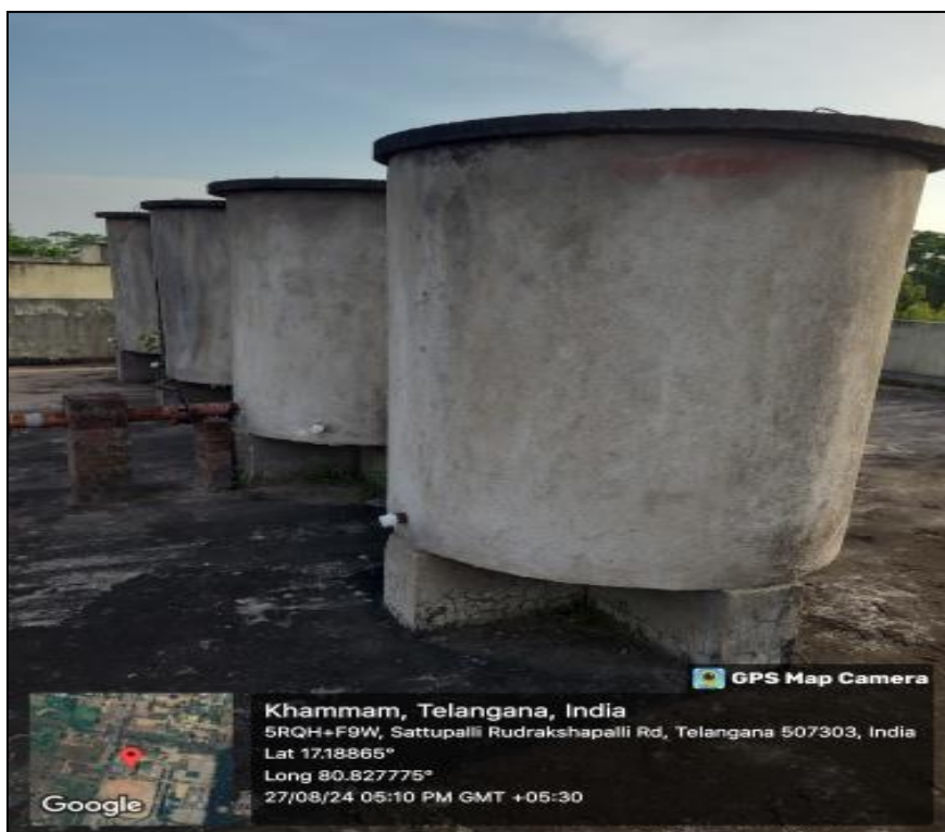
Fig.2.3: Water storage tank in the campus
